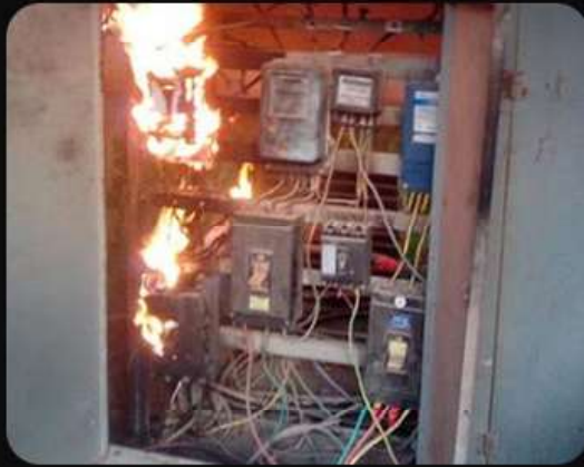
Aging electrical circuits
