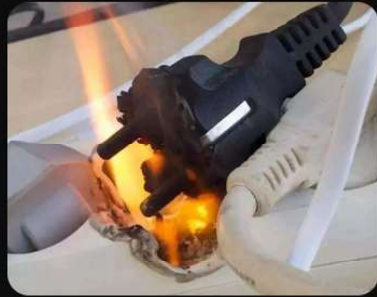
Poor electrical contact
